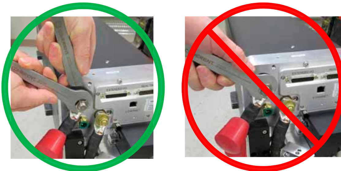
Figure 4-17. +48 VDC Location and Using Two Wrenches
